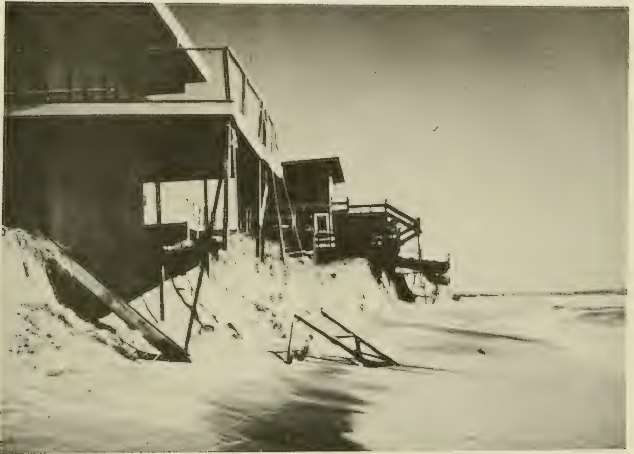
Figure 1-11. Undermining of structures by storm waves, Potham Beach, Maine.
